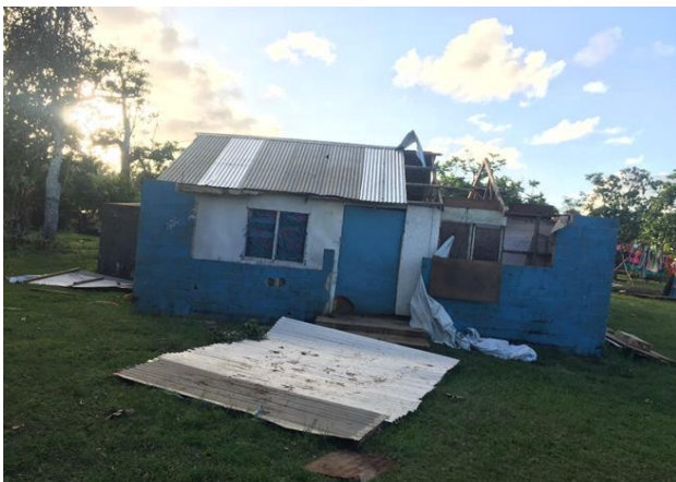
A house damaged by the cyclone in Tongatapu
