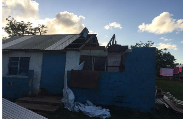
Damaged house in 'Atataa island
