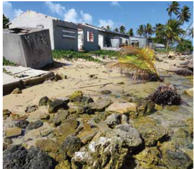
Damaged coastline and houses, Lifuka, Tonga, March 2012.
